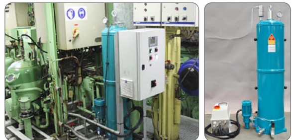
Installed CJC™ Oil Care System 27/108
