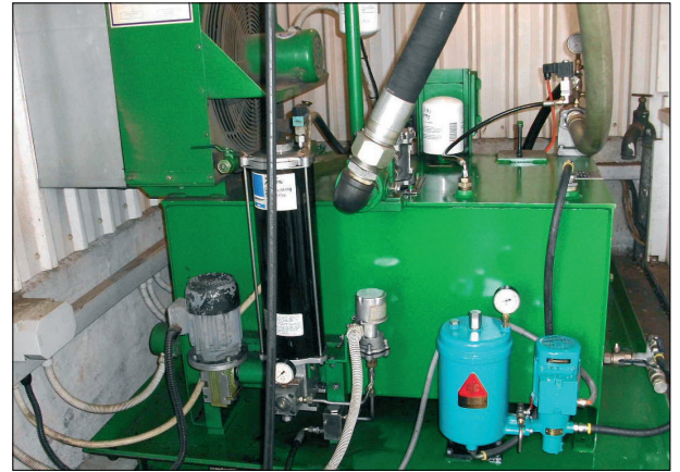
The Hydraulic Power Pack at Taranaki Pine, New Zealand with the CJC™ Fine Filter unit 15/25 installed
