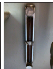
Sight glass - BEFORE fine filtration
