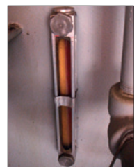
Sight glass - AFTER fine filtration with CJC®
