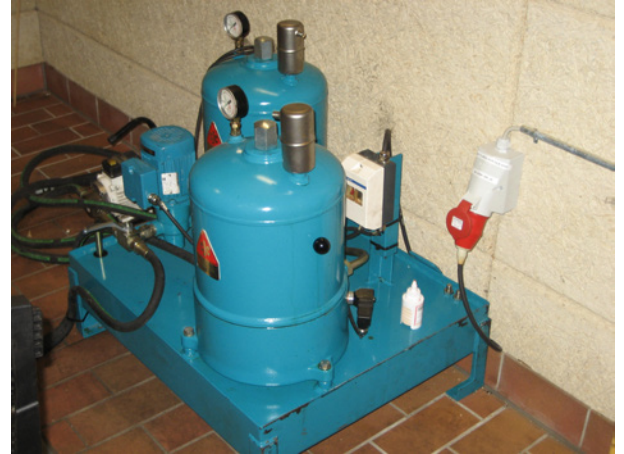
E.ON Danmark A/S, MAN Gas Engine and the CJC® Fluid Treatment unit 27/27-27/27
